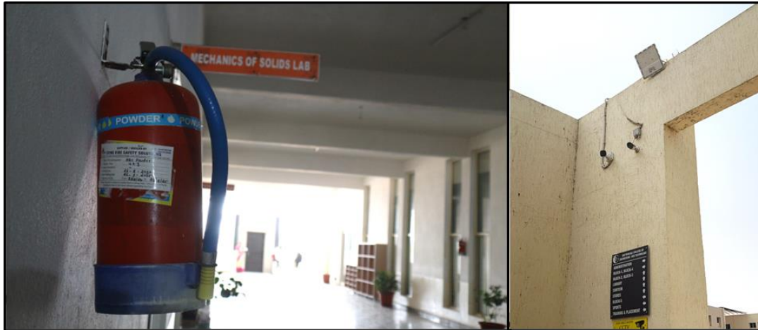
Fire extinguisher and CCTV Surveillance facilities available in the buildings.
