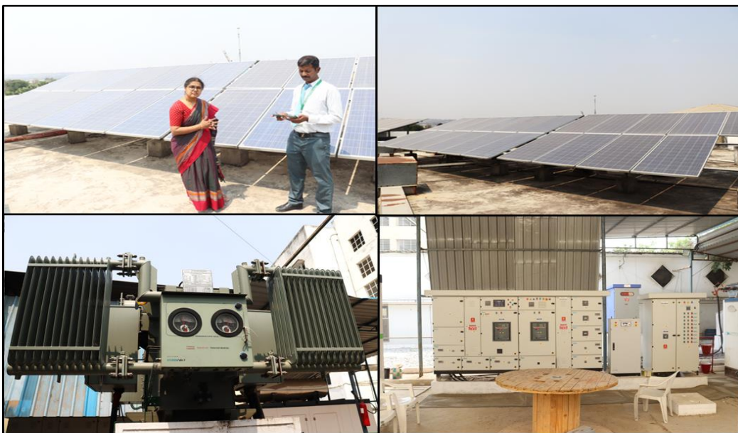
Energy conservation facilities observed in the Campus
